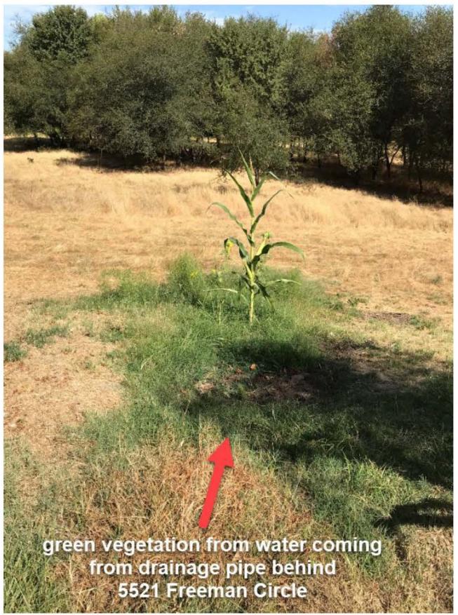
Water from drainage pipe behind 5521 Freeman Circle exiting onto College property at end of summer
