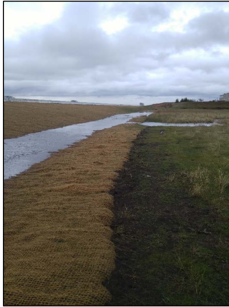
Description: Newly constructed drainage in the Orchard Creek Preserve Date: January 6, 2016 Photographer: Meredith Branstad
